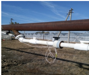
Fig. 7. Appearance of geothermal water supply pipe and device with electronic components installed on it
